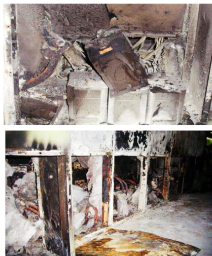
Figure 1: Damage to the voltage transformer.
